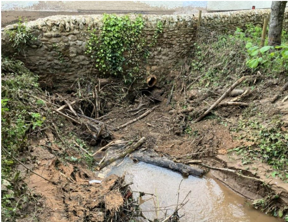
Figure 4.22 DCC Flood Recon photo showing Higher Way culvert on 10 May 2023 partially blocked even after significant clearance works
