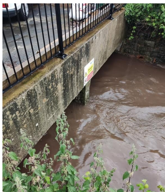
Figure 4.27. Northbrook watercourse entering the culvert underneath Honiton Road can be seen to still have some capacity during the flood event (Photo DCC)
