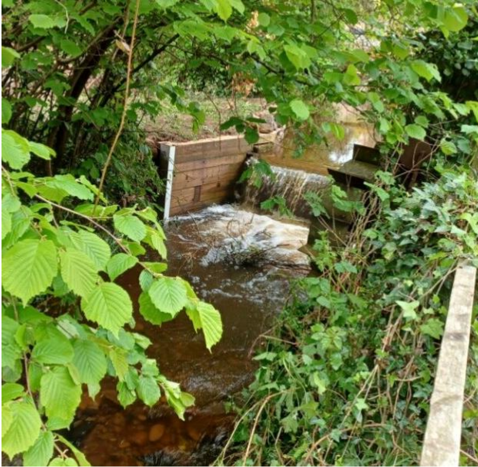
Figure 4.19 DCC Flood recon photo showing weir structure upstream of Exmouth Road, Colaton Raleigh
