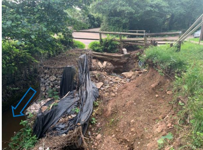
Figure 4.24. EA Flood recon photo showing damage to watercourse and existing gabions at Stoneyford with blue arrow showing flow path
