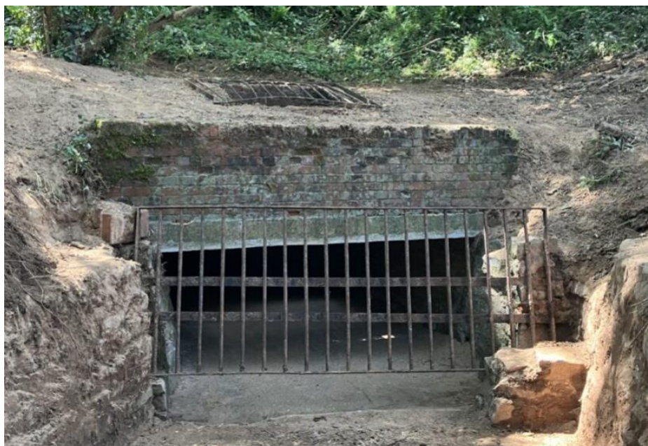
Figure 4.12 - Sidmouth Road culvert inlet in Tipton St John pictured following DCC clearance of structure which had been completely buried in fine sediment and woody material following the 9 th May event, DCC recon photo.
