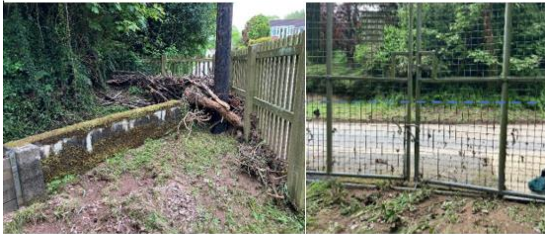
Figures 4.10 and 4.11 Photo on left shows woody debris sat above the culvert inlet, post event. Photo on right shows access gate with padlock which had been forced open assumed due to the force of floodwater impounded by woody debris, both taken by EA during flood reconnaissance.
