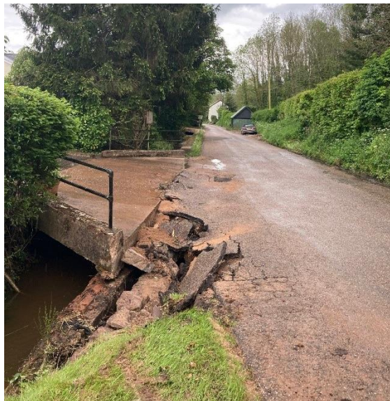
Figure 4.13 EA recon photo showing damage to the public highway along Brookvale at one of many points where flows came out of bank joining existing flows along the road network.
