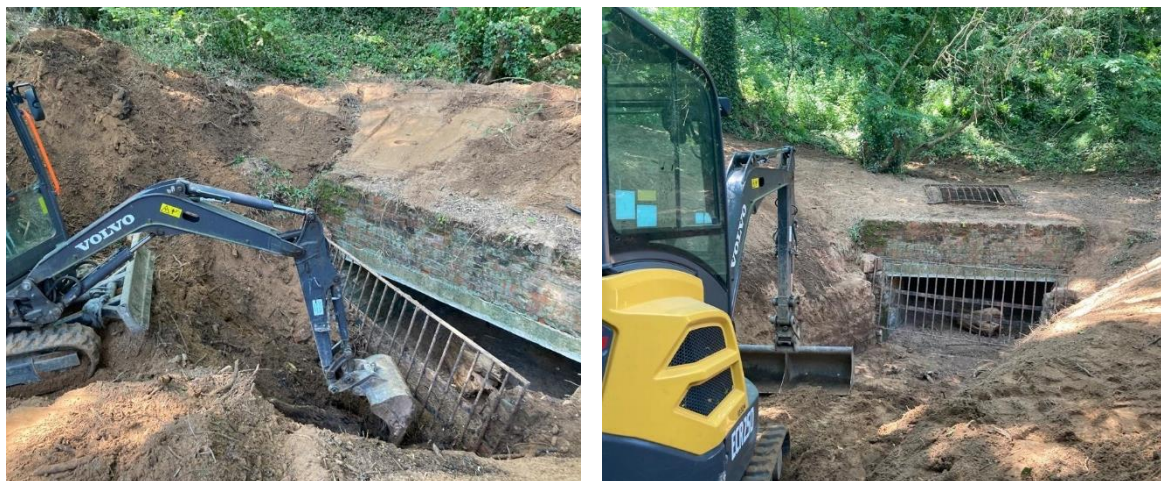
Figure 3.7 Clearance works at Tipton St John Sidmouth Rd culvert (Photo from DCC contractor)
