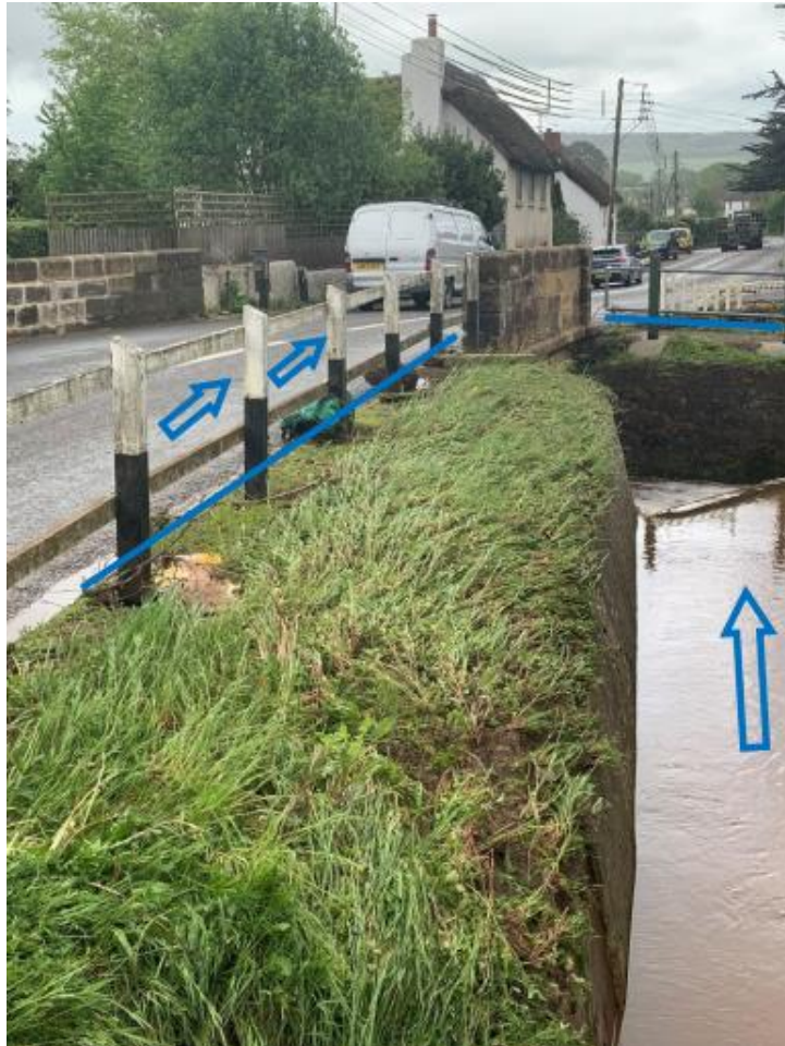
Figure 4.8. EA recon photo showing flow paths marked by blue arrows and water levels marked by blue line at Burrow Bridge where it passes beneath the A3052, structure had inadequate capacity to cope with the May 9 th event.
